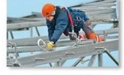
Work at height
