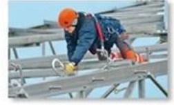
Work at height
