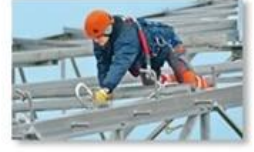
Work at height
