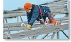
Work at height
