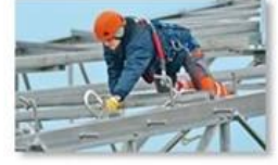
Work at height
