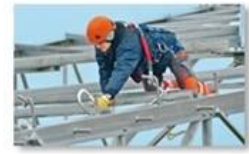
Work at height
