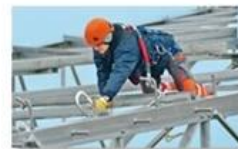
Work at height
