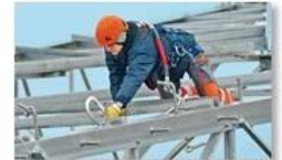
Work at height
