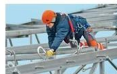
Work at height
