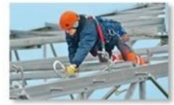
Work at height
