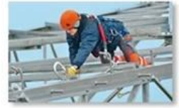
Work at height
