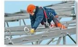
Work at height
