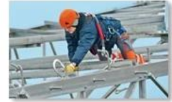
Work at height
