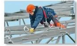
Work at height
