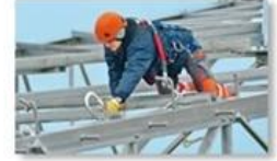
Work at height
