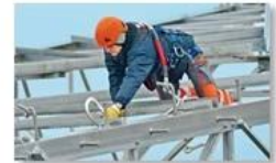
Work at height
