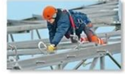
Work at height
