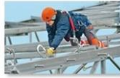
Work at height
