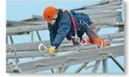
Work at height
