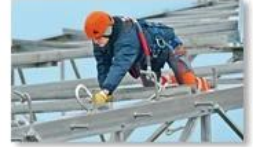
Work at height
