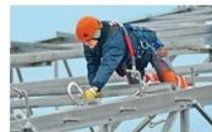
Work at height
