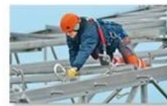
Work at height
