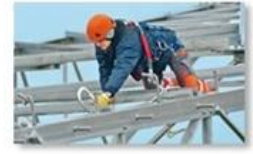
Work at height
