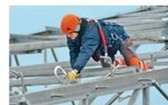
Work at height
