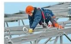
Work at height
