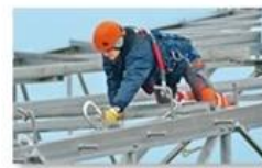
Work at height
