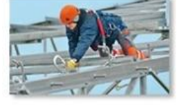
Work at height
