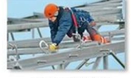
Work at height
