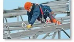
Work at height
