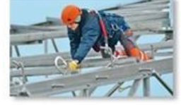
Work at height
