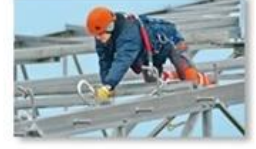
Work at height
