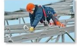
Work at height
